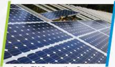
Solar PV Generation System
