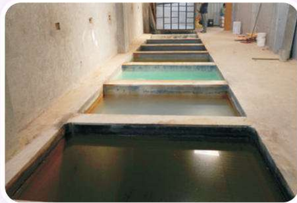
8 Tank Chemical Process
