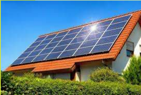
On Grid / Off Grid Solar PV Rooftop (KW/MW)
